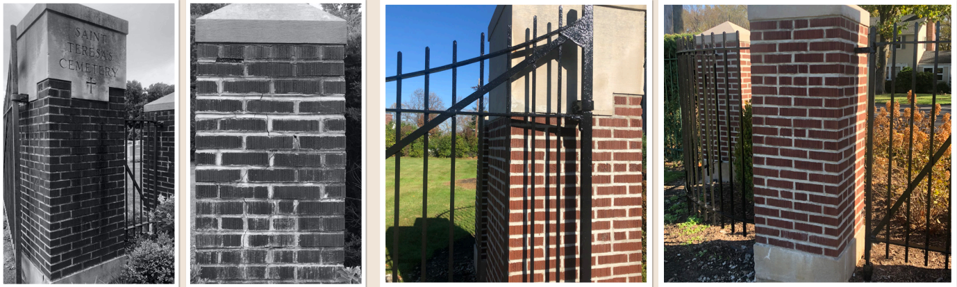
The cemetery columns have been repainted and the gates repainted, the results give a fresh, new appearance to the entrance.
